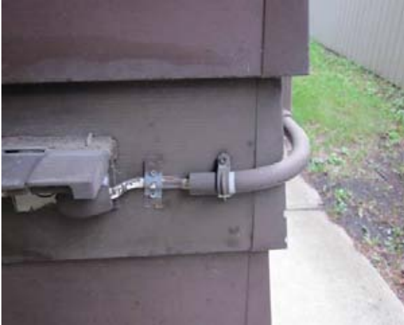
Suspect wiring noted. Contact electrician to evaluate and repair as required to reduce associated hazards.
