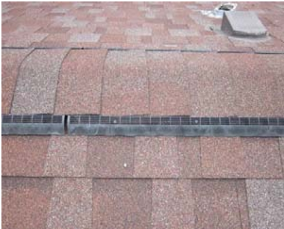
Vents caps noted
